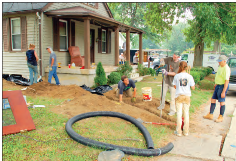
Volunteers from Good Neighbors Home Repair work on exterior repairs at the home of a low-income Chester County resident.
