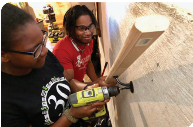
Rebuilding Together Philadelphia construction students repair deteriorating homes to allow low-income, senior homeowners to age in place.
